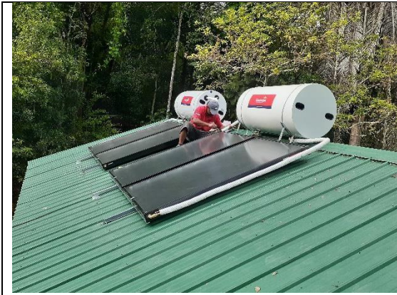
Double system 160-gal Thermosiphon
