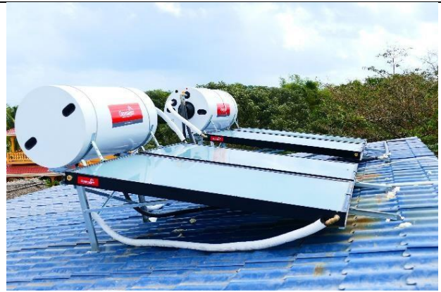
Double system 160-gal Thermosiphon
